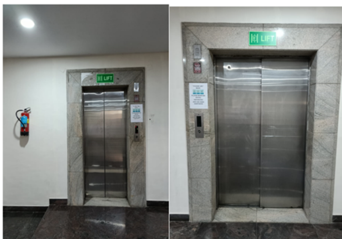
Figure 6.24: Lift facility for staff and students
